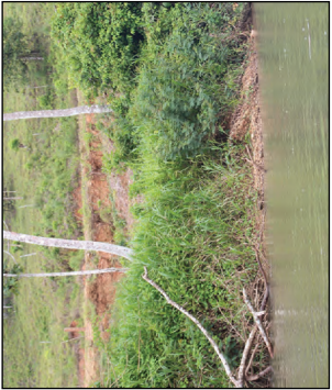
Photo 1. Road fill landslide eroding directly into the river (from boat, May 2012).
