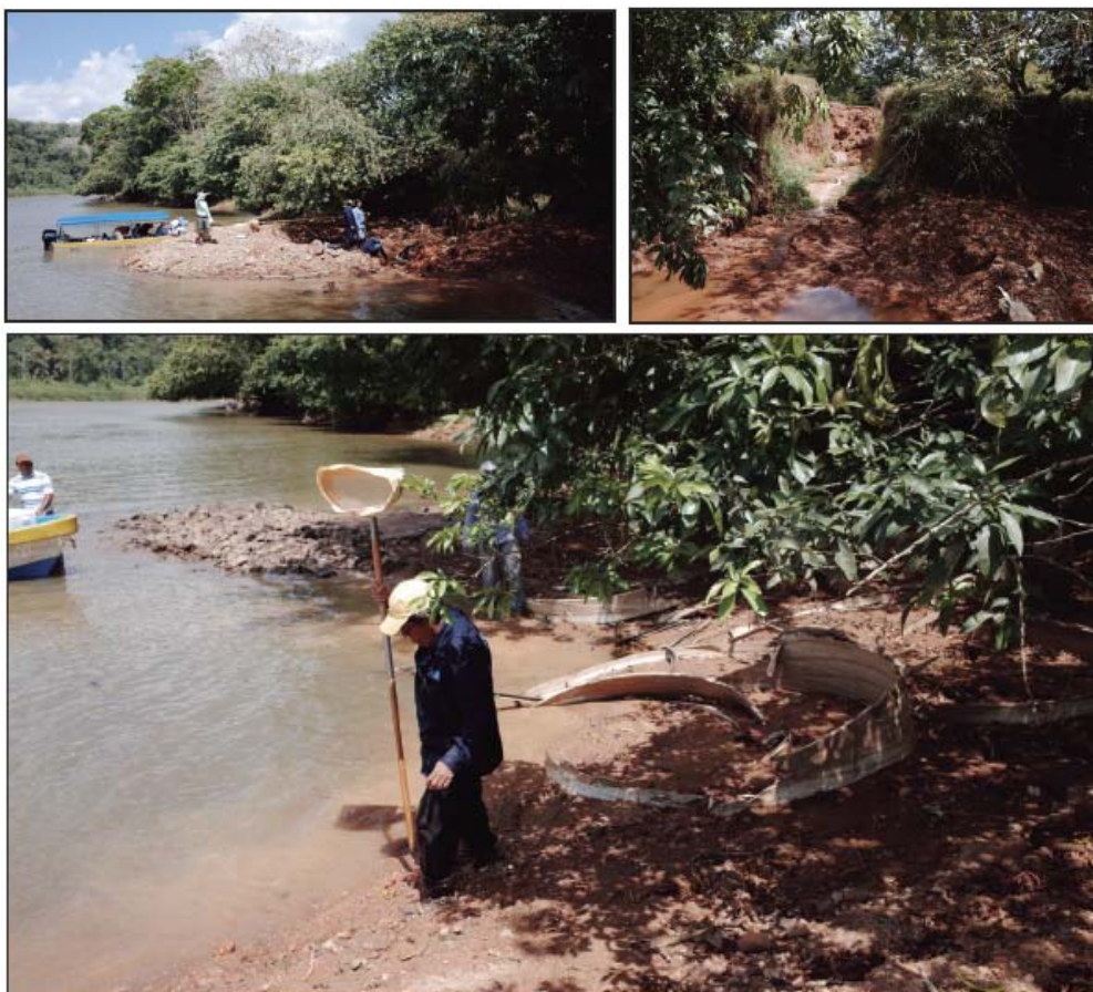
Figure 25. Photographs from a field visit in March 2014 show a delta of sediment with pieces of the failed culvert extending into Río San Juan. New fill material was placed in the channel to partially fill the void created by the failure, but no new culvert was installed.
