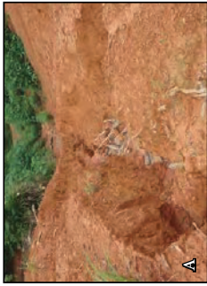
Deep gully on sidecast fill slope (from Mende & Astorga 2013, p40). View down the gully to Rio San Juan.
