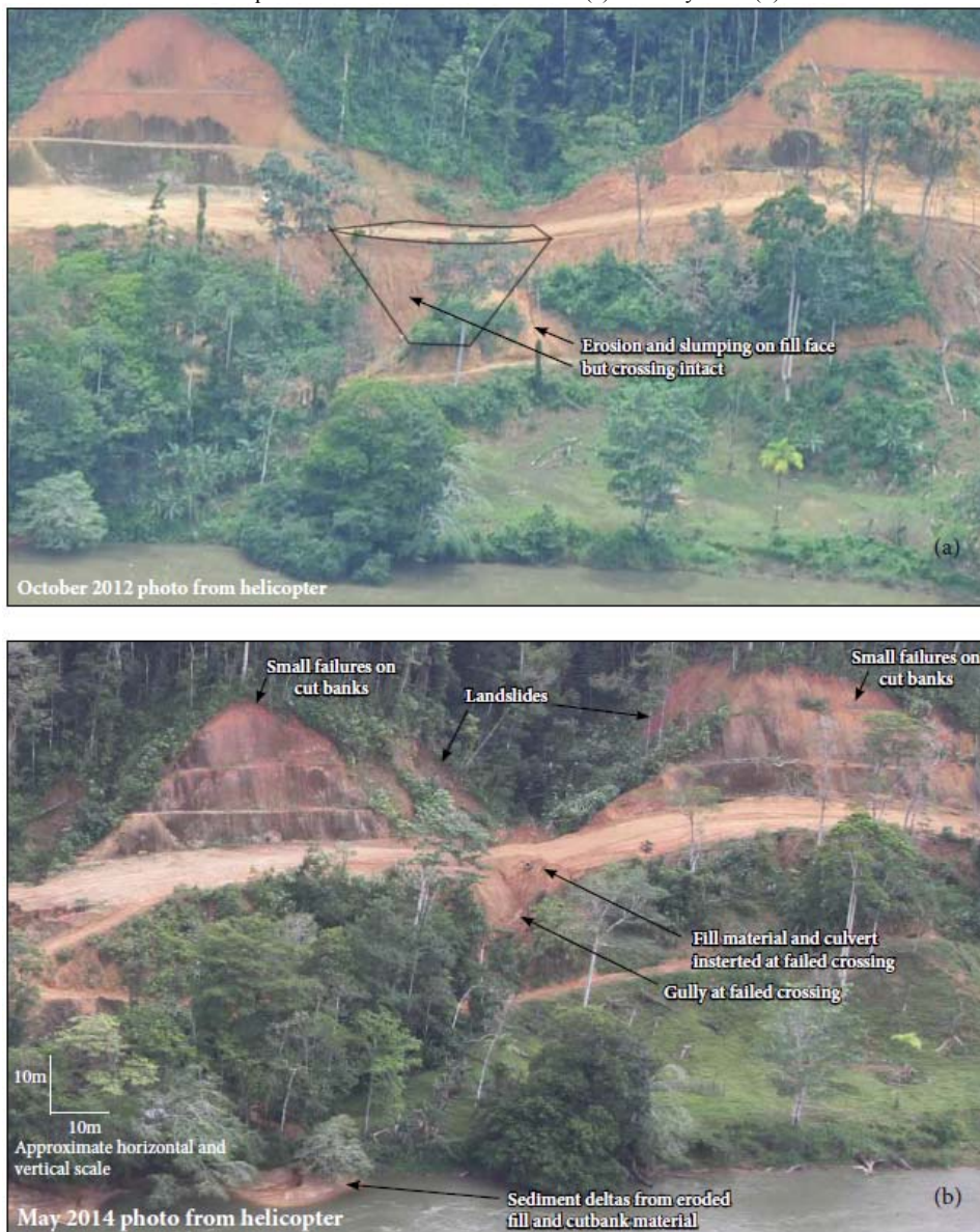
Figure 13. Eroding Site 9.5, 18.1 km downstream of Mojon II. Oblique aerial views from October 2012 (a) and May 2014 (b).
