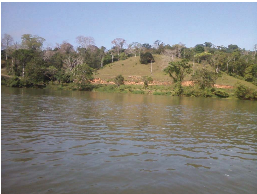
PHOTO 9 - Location: RKM 2.5 (from boat, May 2014). This section of the Route was constructed by cutting into the toe of existing slope that is very close to the bank of the San Juan River. The cut that was constructed into the hill is too steep and unprotected. The steep cut slope and the nature of the unprotected slope located at the toe of a fairly high hill will promote erosion as water will flow over the cut during periods of precipitation that will continue to cut the slope and produce sediments that will wash into the San Juan River.
