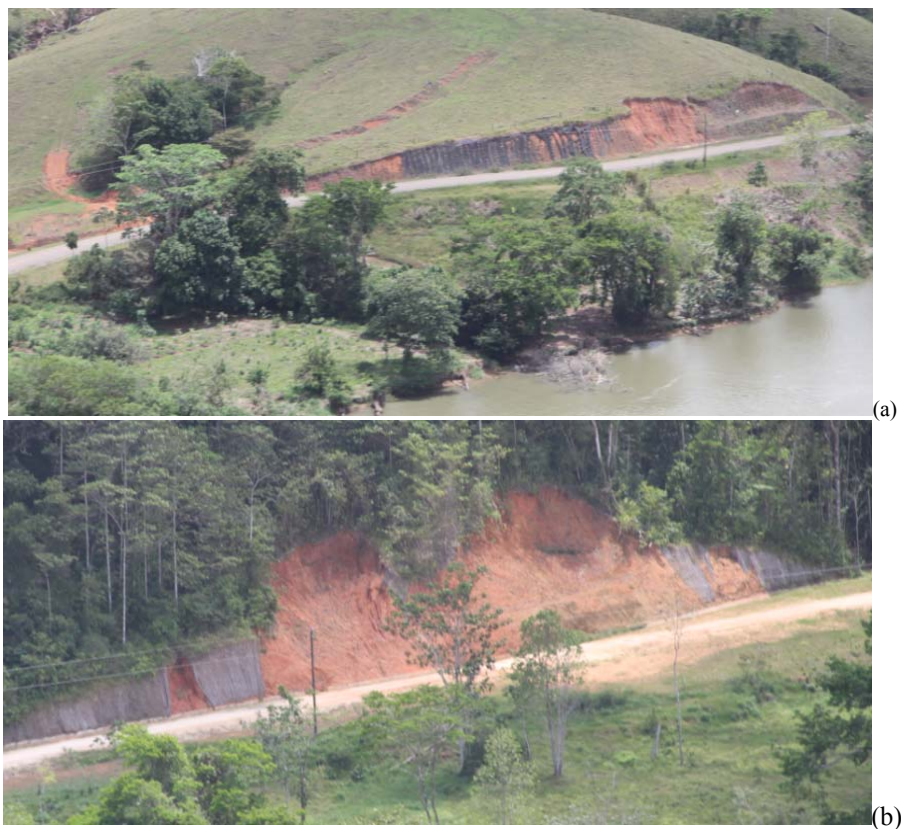
Figure 27. Failing black plastic erosion control fabric approximately (a) 6.8 km and (b) 10.0 km downstream from Mojon II, respectively.
