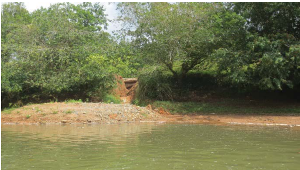
PHOTO 3 - Location: RKM 20.3 (from boat, May 2014). Road section with improper stream crossing consisting of a log bridge that has resulted in constricted of water flow and the creation of sediment delta in the River.
