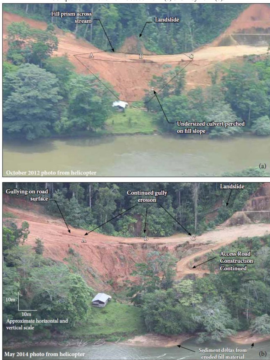
Figure 15. Eroding Site 9.6, 18.2 km downstream of Mojon II. Oblique aerial views from October 2012 (a) and May 2014 (b).
