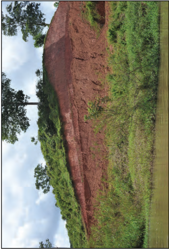
Photo 2. Eroding cutslope within close proximity to the river (view from riverboat, October 2012).
