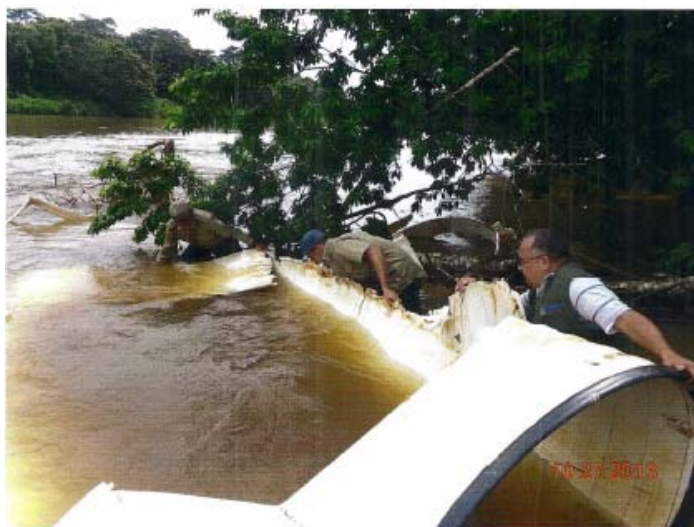
Figure 12. Nicaraguan staff working in delta prograding into Río San Juan to remove plastic pipe washed out of stream crossing fill at Eroding Site 9.4. Photograph date: October 27, 2013. Provided by the Government of Nicaragua.
