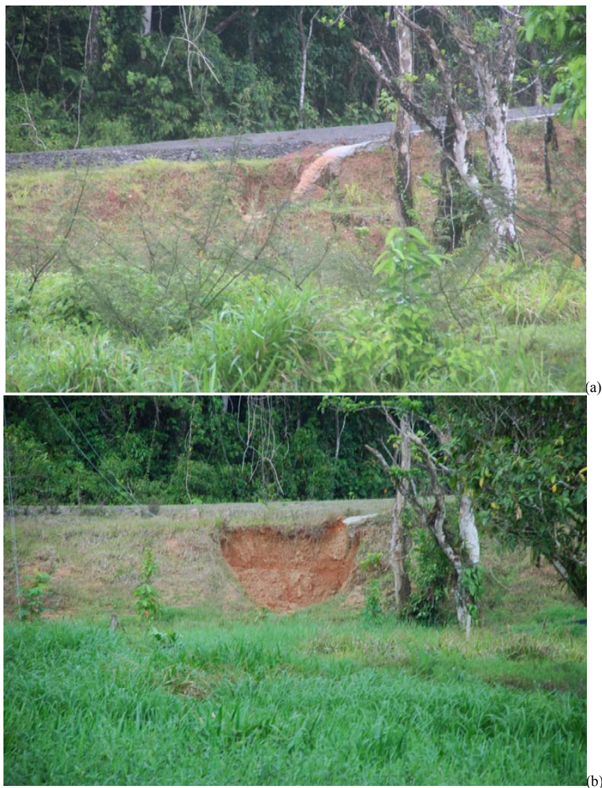
Figure 26. Photo of road runoff directed from drainage structure into fill in May 2013 (a), and resulting erosion in May 2014 (b).
