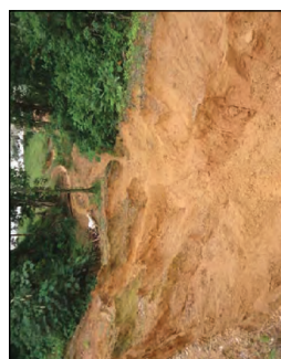
Photo 2. Eroding fill prism with drainage path leading to river (from Mende & Astorga 2013, p43).
