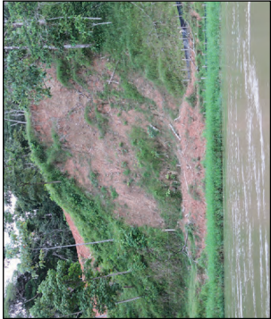
Photo 1 Steep eroding slope of sidecast fill material and deposits along toe of slope. (view from riverboat, October 2013).
