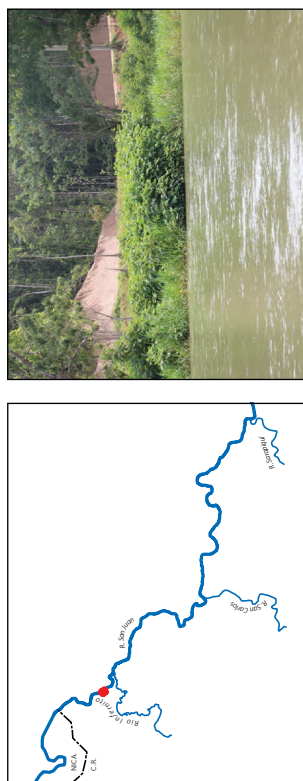
Photo 1. Eroding road cuts and fill slope in close proximity to the river (view from riverboat, May 2013).
