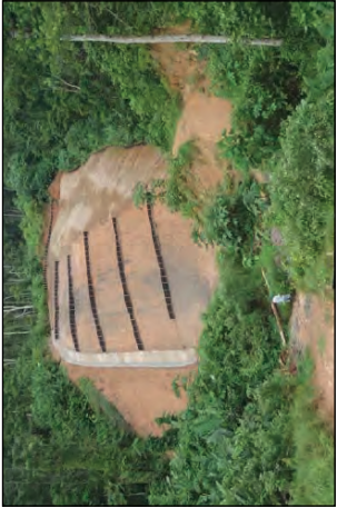
Photo 1. Gully through road and pioneered but incomplete road cut through steep terrain (from Mende & Astorga 2013, p38).
