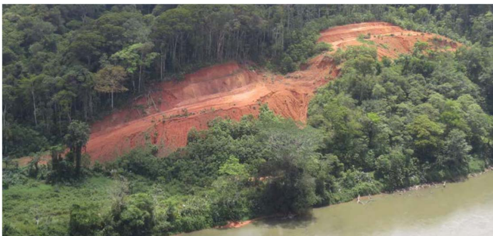
PHOTO 4 - Location: RKM 16.1 to 16.5 (from helicopter, May 2014). Steep cuts and slopes were constructed in these erodible soils at slopes that are not generally considered stable or recommended for these types of soils. Lack of planning, design and mitigation measures have all led to the conditions observed.
