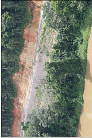
Photo 2. Steep cut and fill slopes (view from helicopter, October 2013)
