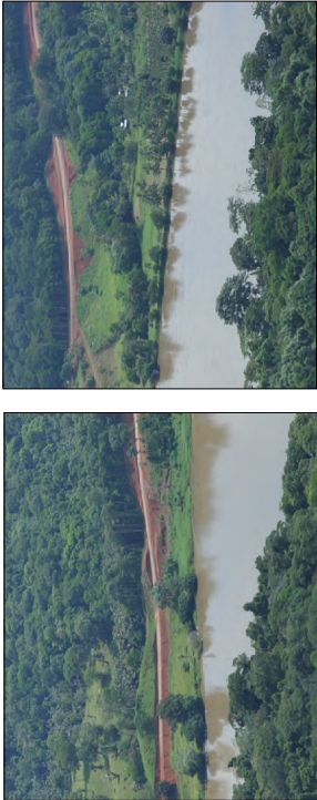
Photo 1. Gullying fill slopes (view from helicopter, October 2012).
