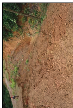
Photo 1. Eroding fill prism placed across drainage path (from Mende & Astorga 2013, p43).
