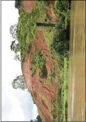
Photo 1. Eroding cutslope within close proximity to the river (view from riverboat, October 2013).
