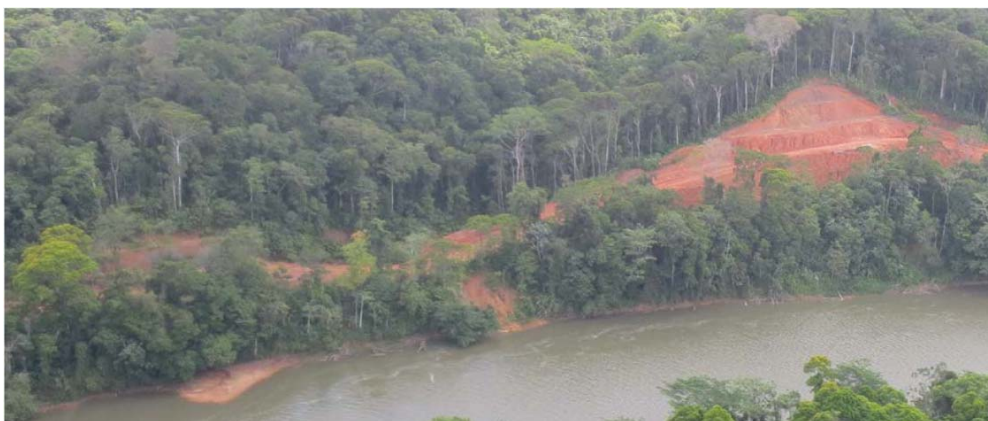
PHOTO 8 - Location: RKM 18.3 to 18.6 (from helicopter, May 2014). The relationship between topography and the management of storm water not properly managed has resulted in significant erosion. Earthwork activities employed to construct the roadway have resulted in exaction into steep slopes (due to the lack of appropriate route selection and design) to accommodate the roadway in steep terrain. The construction of roadways in steep topography has resulted in the acceleration of water moving over exposed soils, further resulting in erosion and sediment loading as a direct impact to San Juan River.
