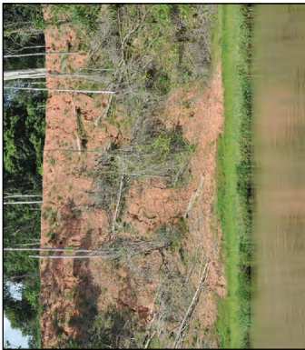
Photo 2 Steep eroding slope of sidecast fill material and deposits along toe of slope. (view from riverboat, October 2012).
