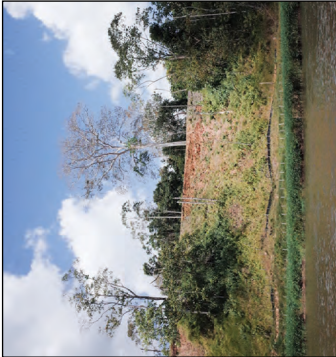
Photo 3 Steep eroding slope of sidecast fill material, overwheeled fill material and deposits along toe of slope. (view from riverboat, March 2013).
