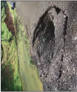
Photo 1. Collapsed road fill sink hole at blocked drainage (from Annex 5, Mende et al 2013).
