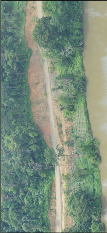
Photo 2. Steep eroding cut and fill slope in ES-01.5. (from helicopter, October 2012).
